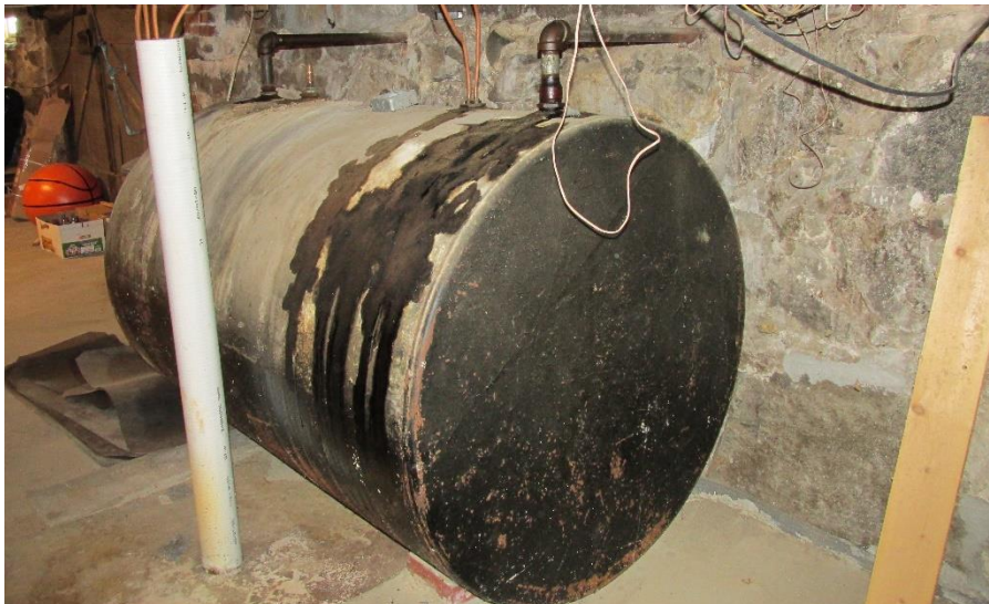
Town Hall - Fuel Oil Tank
