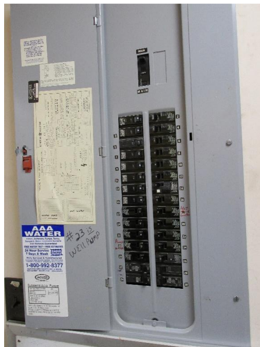
Library Furnace Room - MDP
