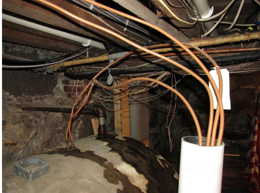
Town Hall - Fuel Oil Piping
