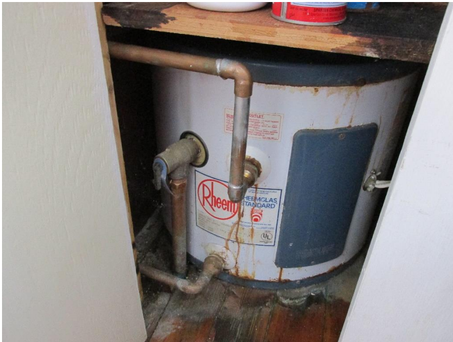
Town Hall Main Floor - Entry Lavatory Water Heater
