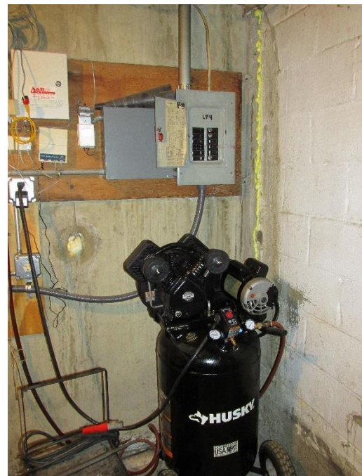
Fire Station - Distribution Panel in Old Boiler Room
