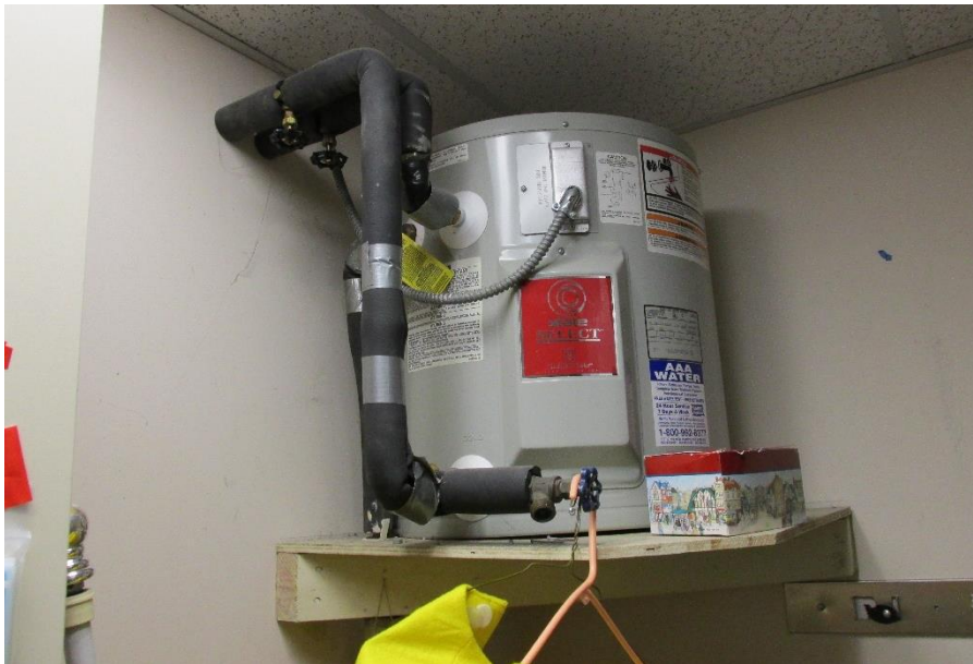
Library Furnace Room - Water Heater
