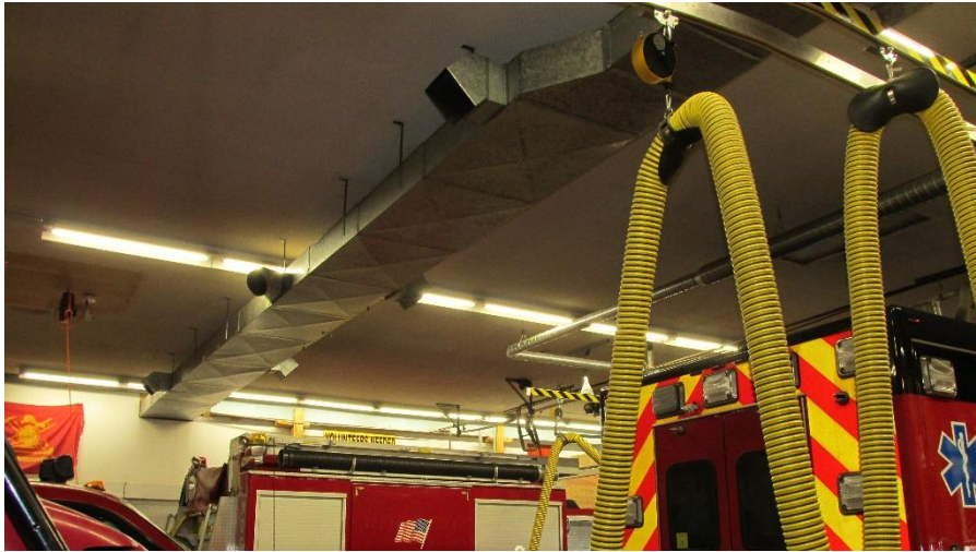
Fire Station Apparatus Room - Abandoned Ductwork
