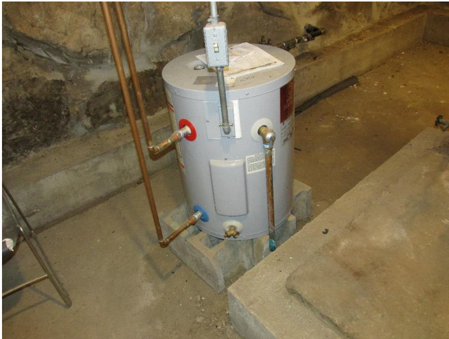
Town Hall Boiler Room - Water Heater in Boiler Room
