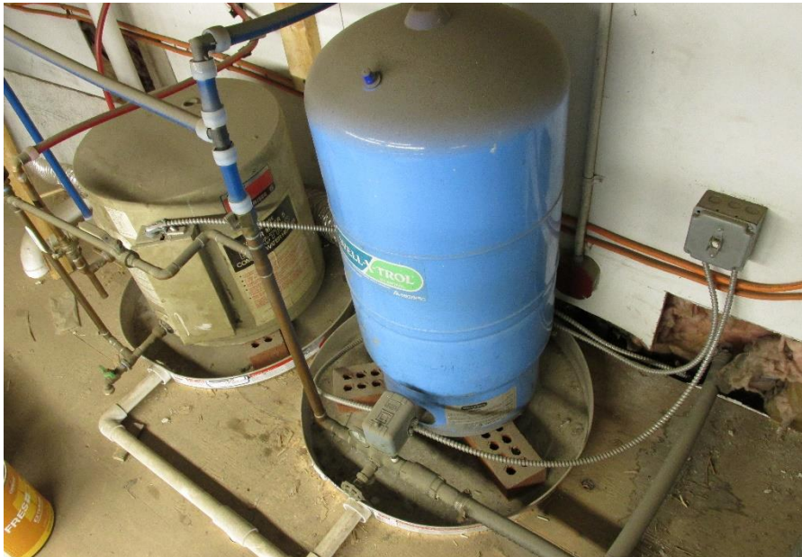
Public Works Mezzanine - Domestic Water Entrance
