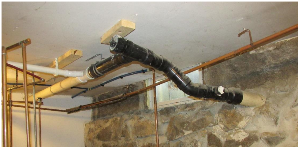
Town Hall Boiler Room - Sanitary Main Exit Rear
