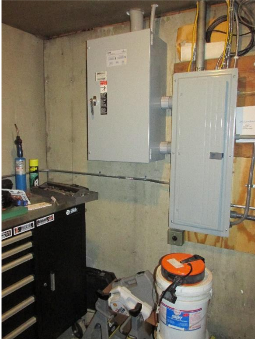
Fire Station - Distribution Panel in Old Boiler Room
