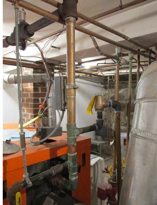
Town Hall Boiler Room - Connections
