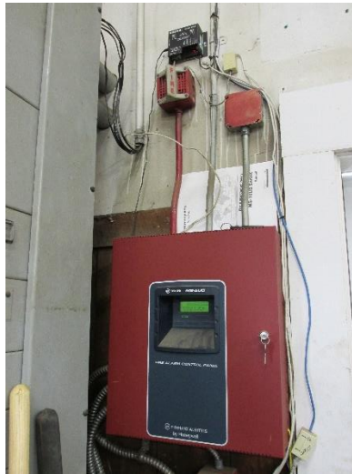
Public Works - Fire Alarm Panel
