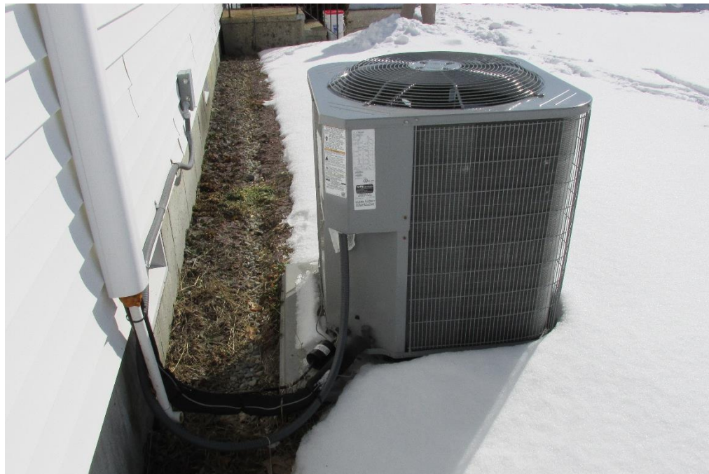
Police Dept Exterior - Air Conditioning Condensing Unit
