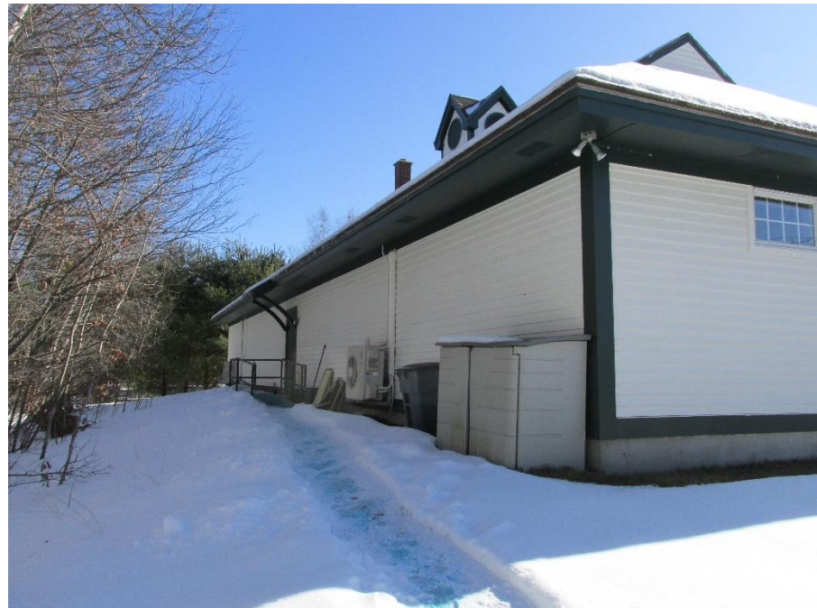
Library Exterior - Heat Pump Outdoor Units
