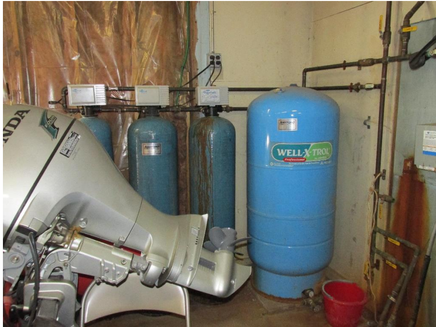
Fire Station – Domestic Water Well Entrance
