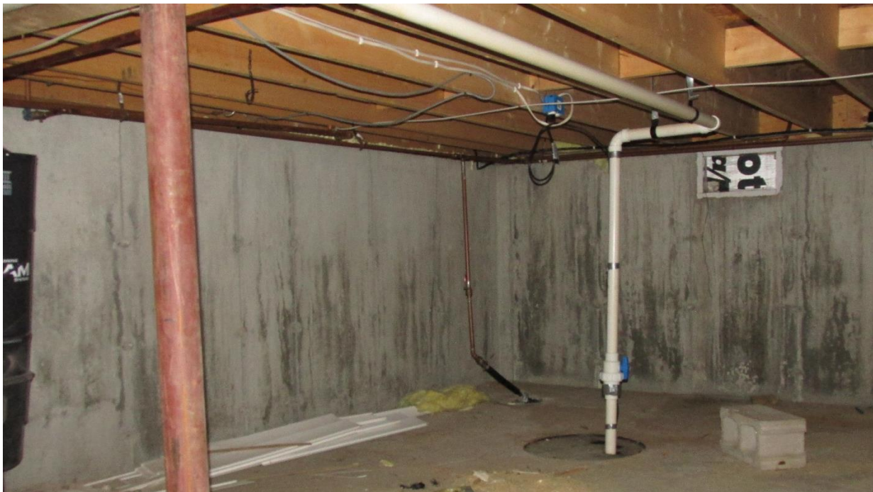
Police Dept Crawl Space - Domestic Water Entrance and Sump Pump
