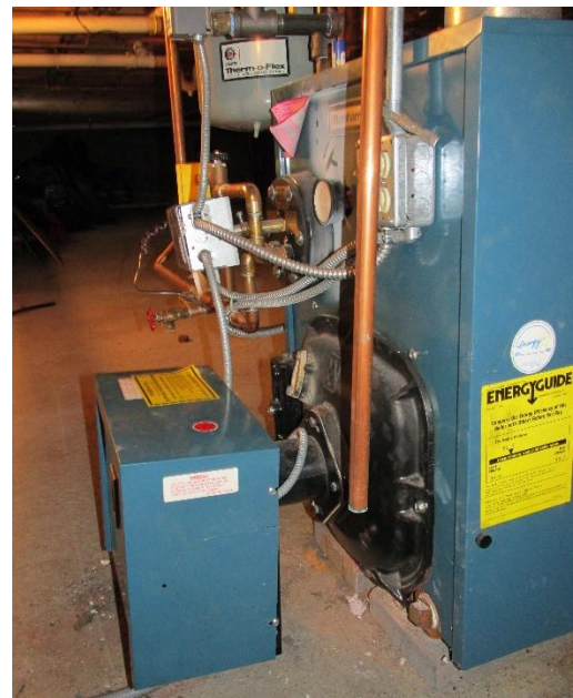
Police Dept Crawl Space - Boiler Front Showing Tankless Coil
