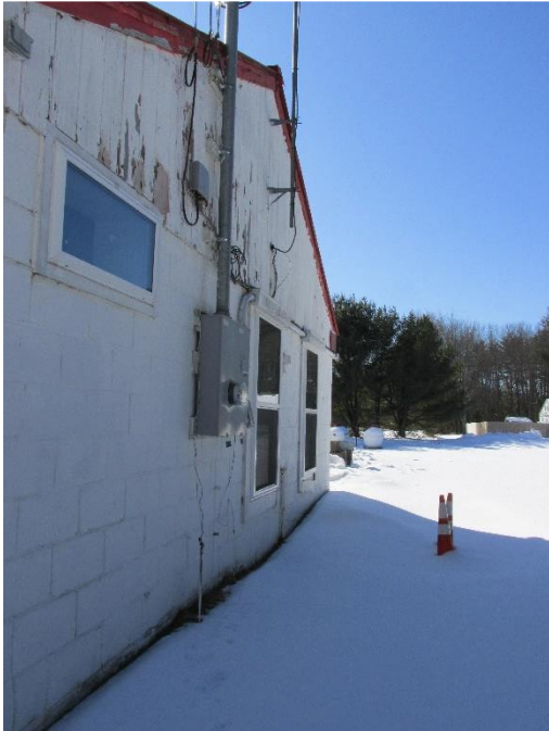
Fire Station - Electric Meter & Conduit to 2nd MDP
