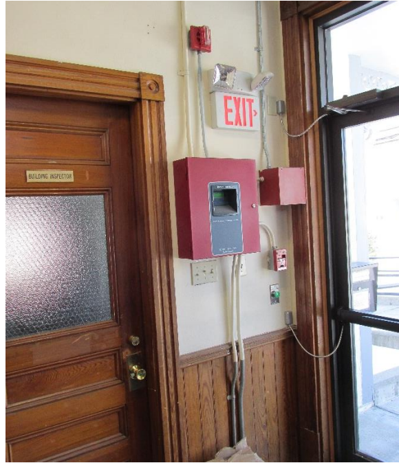
Town Hall - Fire Alarm Panel
