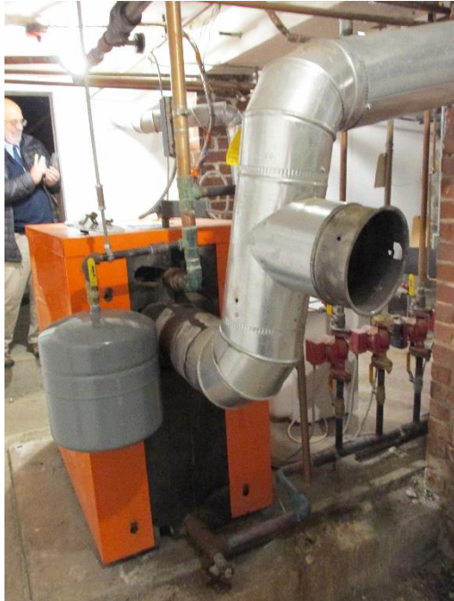
Town Hall Boiler Room - Connections
