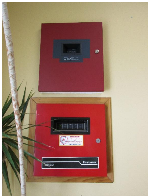
Library Fire Alarm - Fire Alarm Panels
