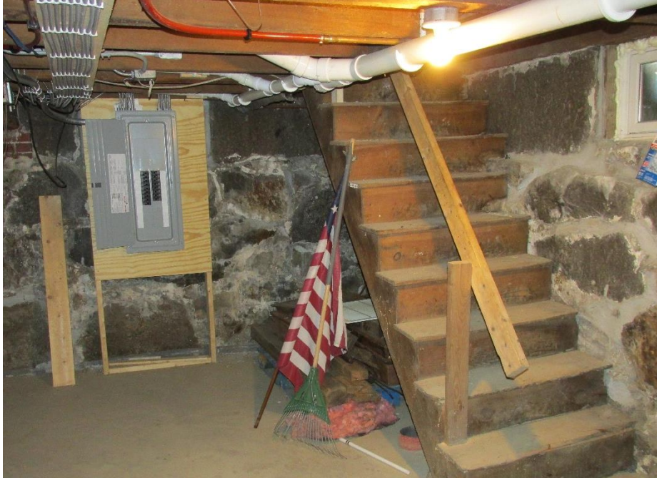
Town Hall Basement – Electrical Distribution Panel in Basement
