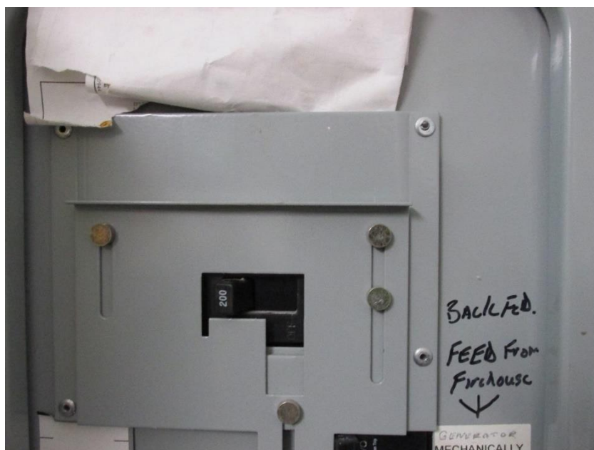
Police Department MDP – Emergency Generator Interlock
