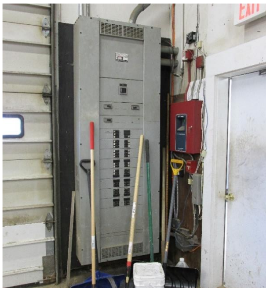
Public Works - Electrical Entrance
