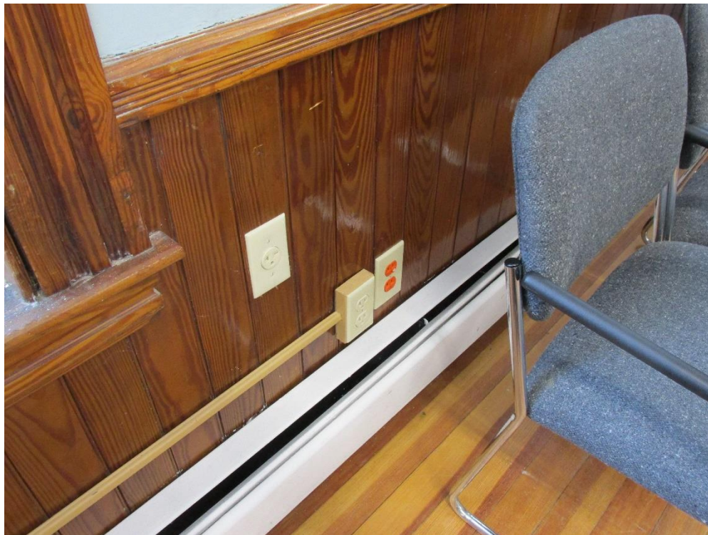
Town Hall Main Floor – Electrical Power Outlets
