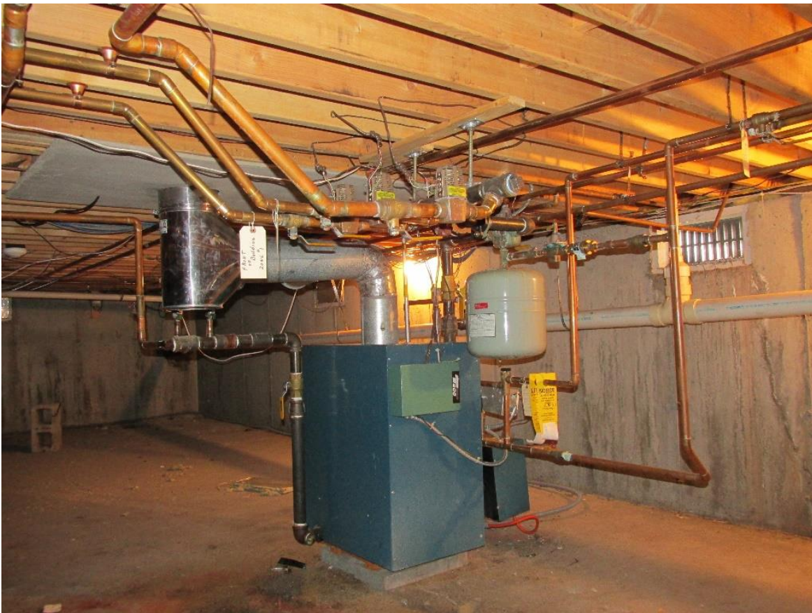
Police Dept Crawl Space - Oil Fired Hot Water Boiler
