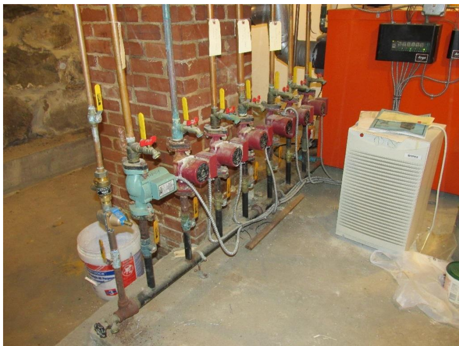
Town Hall Boiler Room - Zone Pumps and Make Up Feed
