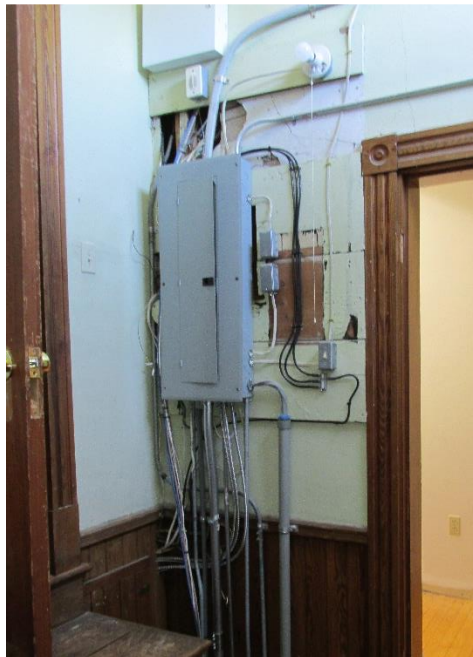
Town Hall Upstairs - MDP on Second Floor Landing, Rear
