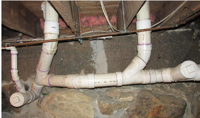
Town Hall Basement - Sanitary Main at Front
