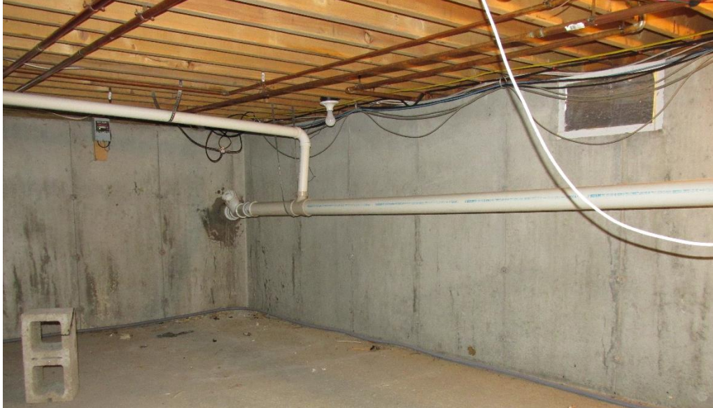
Police Dept Crawl Space - Sanitary Drainage Main
