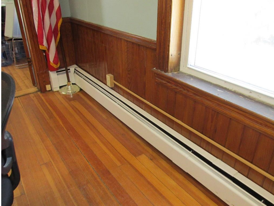
Town Hall Main Floor – Fin Tube Baseboard
