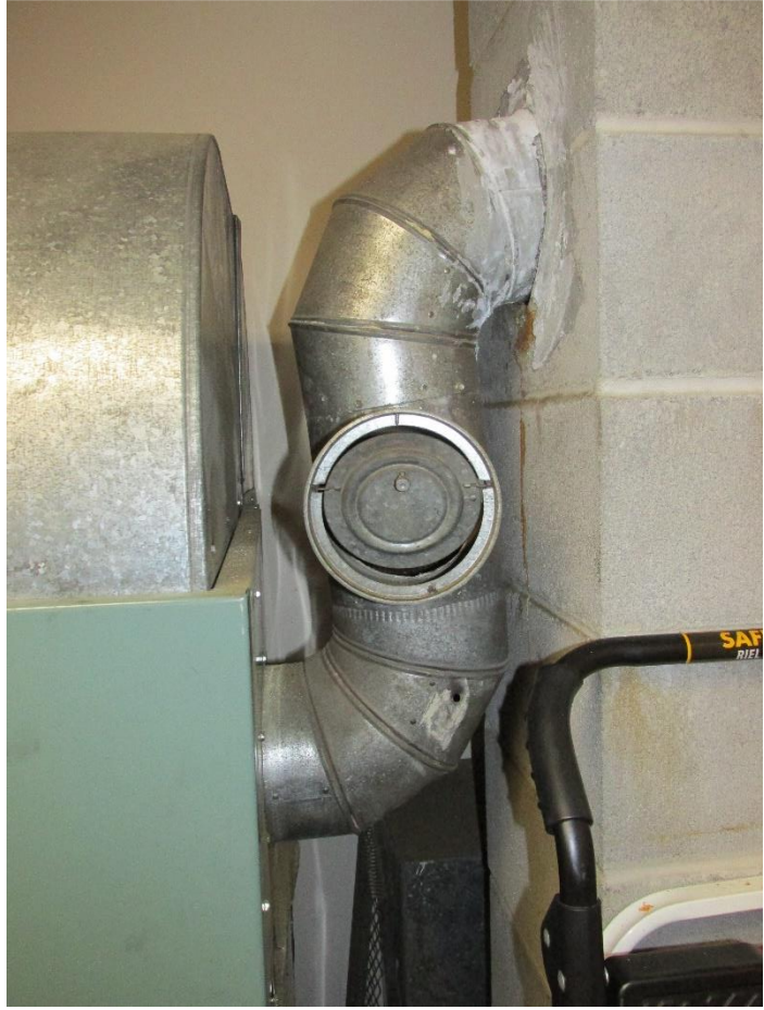
Library - Furnace Flue Pipe Proximity to Return Ductwork
