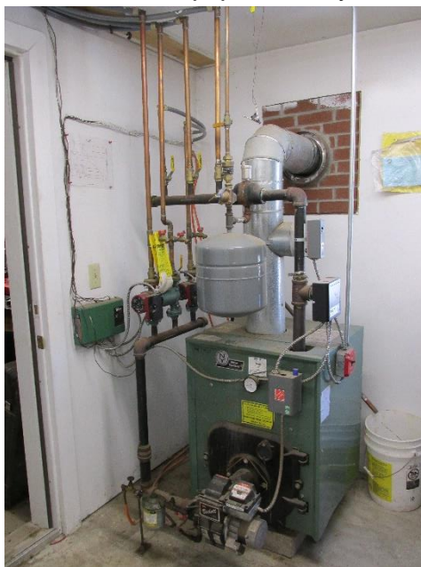
Public Works Boiler Room - Oil-Fired Boiler
