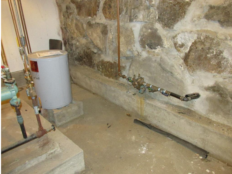
Town Hall Boiler Room - Domestic Water Entrance
