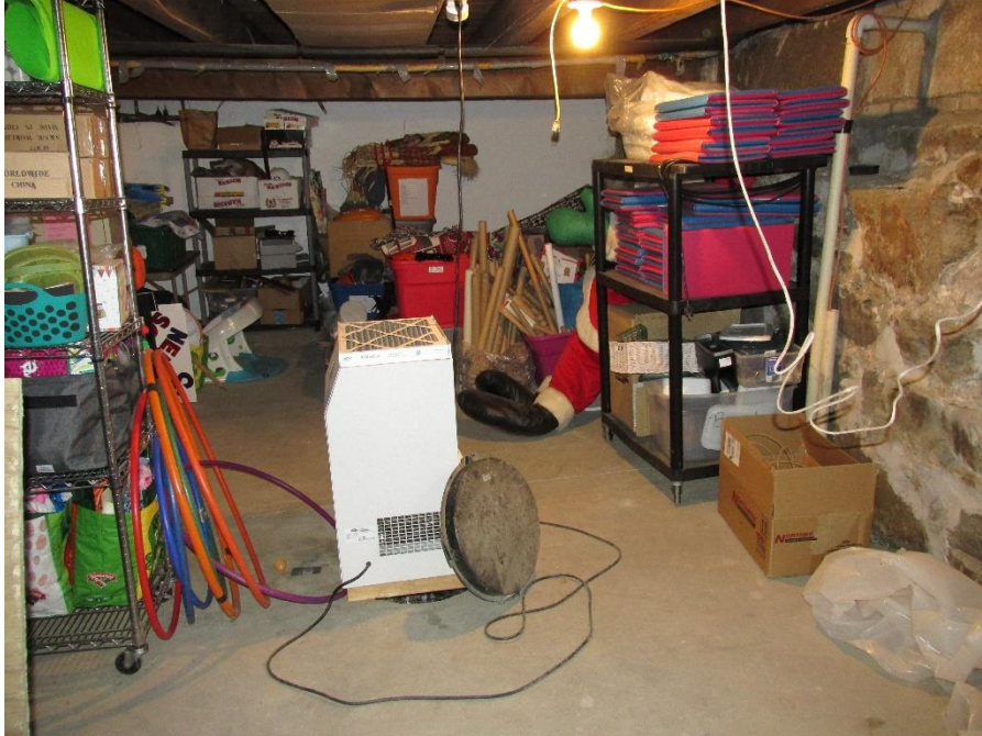
Town Hall Basement - Sump Pump West
