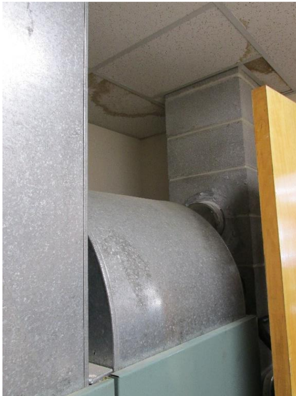
Library - Ductwork at Furnace Uninsulated
