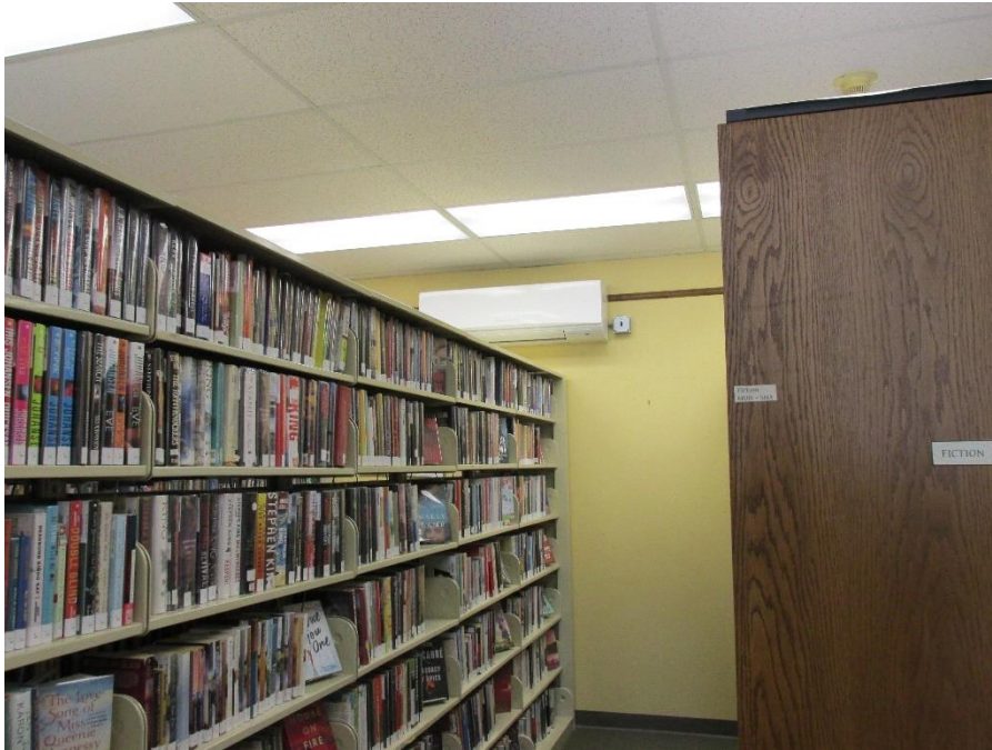
Library Interior - Mini-Split Air Conditioner
