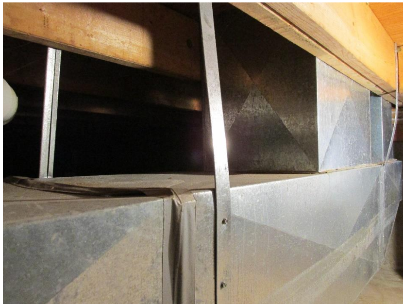
Library Crawl Space - Uninsulated Ductwork
