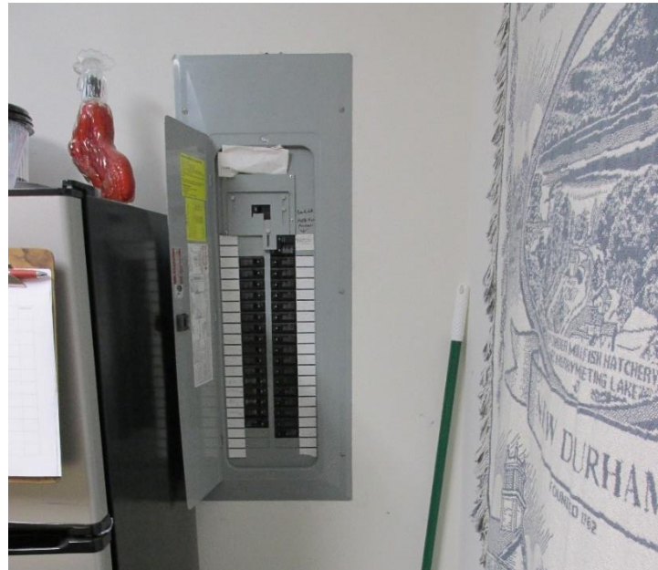
Police Department Electrical - 200A MDP
