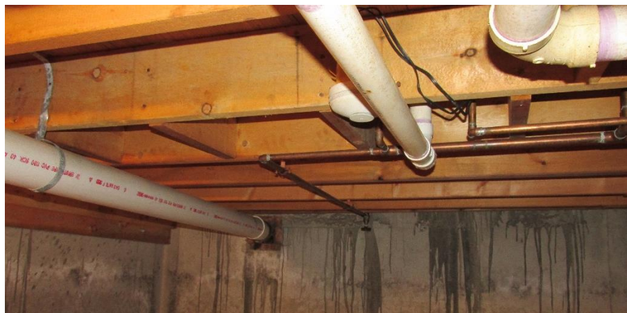
Library Crawl Space - Sanitary Drain
