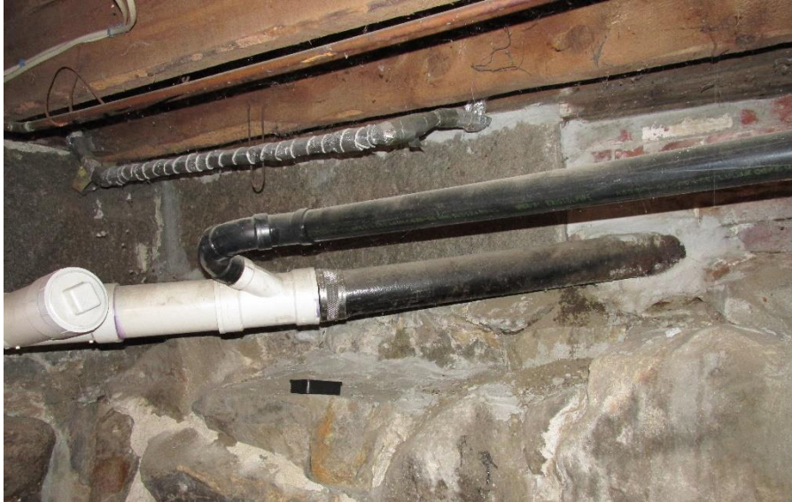
Town Hall Basement - Backward Sanitary Main Fitting
