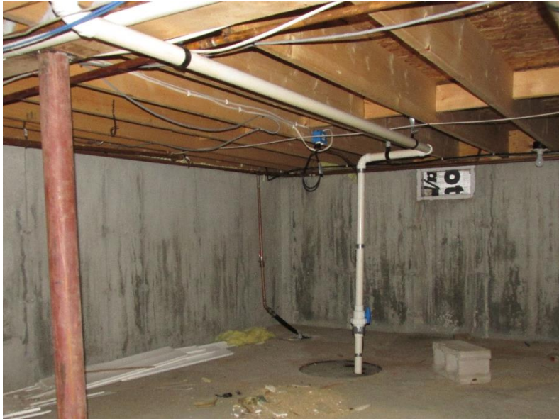
Police Dept Crawl Space - Domestic Water Entrance
