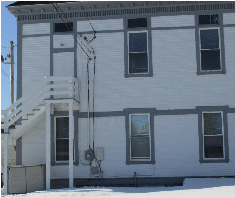
Town Hall Exterior - Electric Meter and Fuel Oil Fill & Vent
