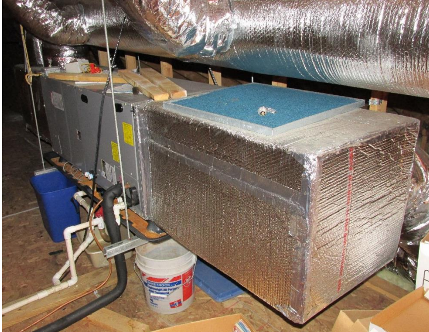
Police Dept HVAC - Air Handler in Attic Space
