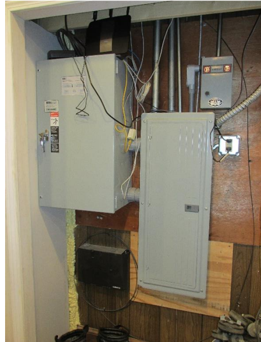
Distribution Panel at Meter w/Gen Tran Switch
