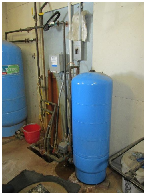
Fire Station Well - Domestic Water Well Entrance
