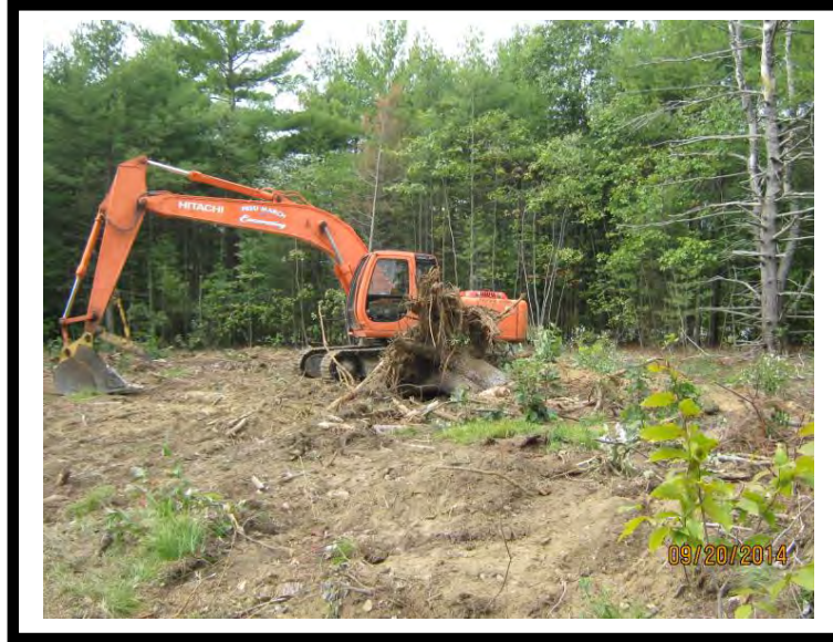
March Excavation clearing the lot for the Boodey House Lot, Located corner of Berry and Stockbridge Corner Roads.
